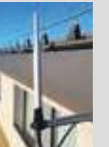
Wi-Fi HaLow™ Access Points Installed in Office Buildings
