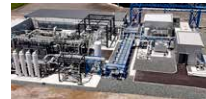
Chita-Midorihamas Works Hydrogen Production Plant (Commenced operations in June 2024)
