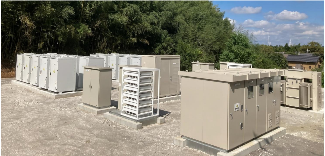
Sanbu District BESS Station in Chiba Prefecture
