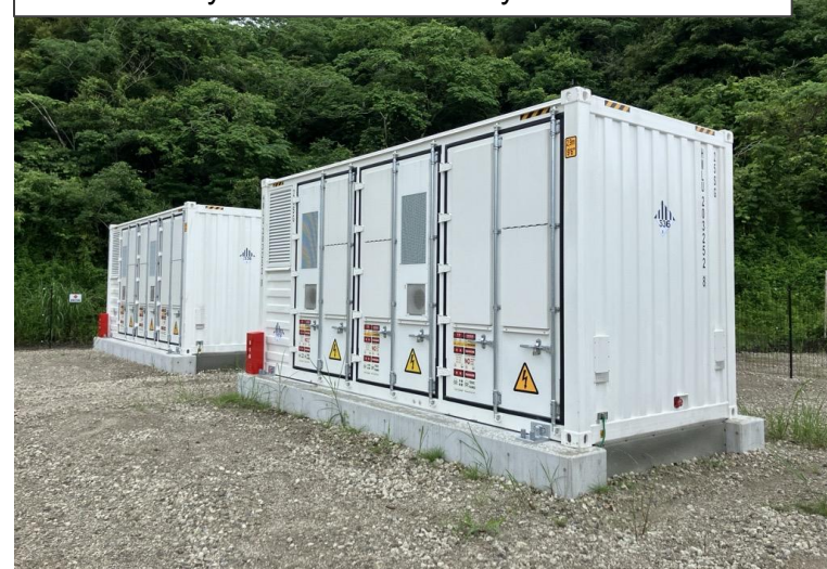
Kushima City BESS Station in Miyazaki Prefecture
