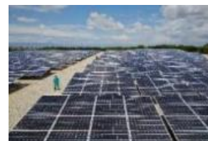
Solar power generation
