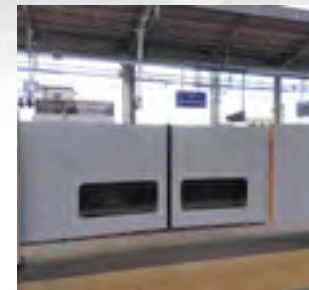
Movable platform gates (Kayashima Station)
