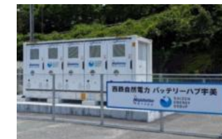
NNR Shizen Energy Battery Hub Umi
