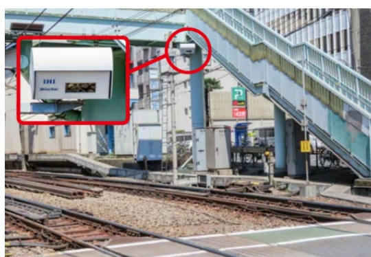
Obstacle detector for railway crossings
