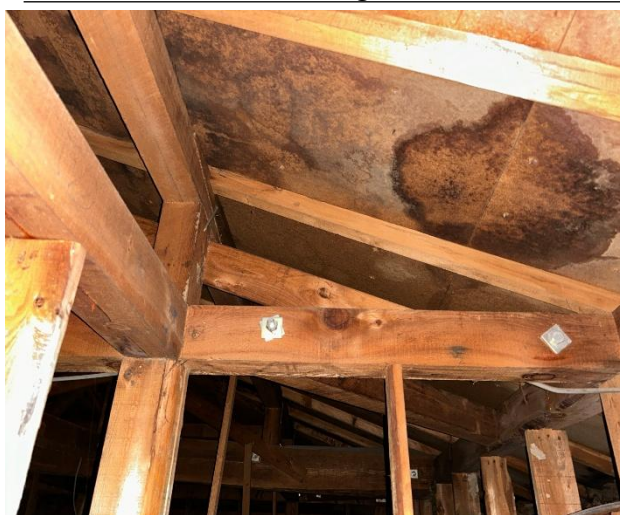
Rain Leakage Risk
