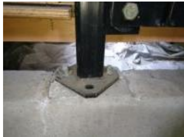
Unstable foundations were discovered after purchasing. This needed to be repaired before sale which led to additional costs.
