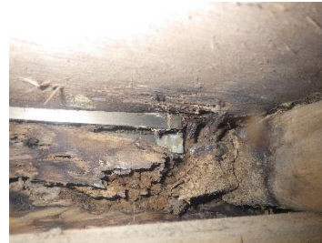
An instance where termite damage was overlooked, resulting in major restoration work including replacement of parts of the wooden structure.
