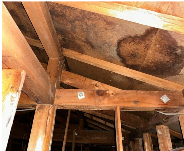
Rain Leakage Risk
