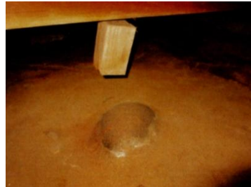
Case in which subsidence under the floor was discovered after purchasing. A major rebuilding of the foundation was necessary.
