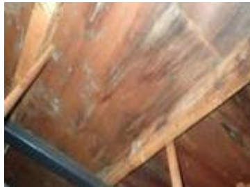
Case in which the roof leaked after sale. A full repair was carried out under the warranty against defects.
