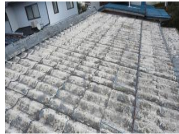
Case in which deterioration in roof materials was noticed after sale. As a partial repair was not possible, the entire roof had to be replaced.
