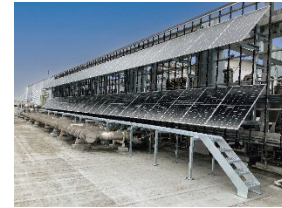
Solar panels on The Keihanshin Fuchu Building
