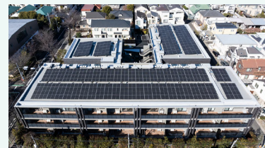
Solar panels installed across the entire rooftop
