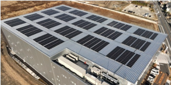
Solar power plant that supplies electricity to I-NET's No. 1 Data Center
