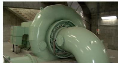
① Hydroelectric power
