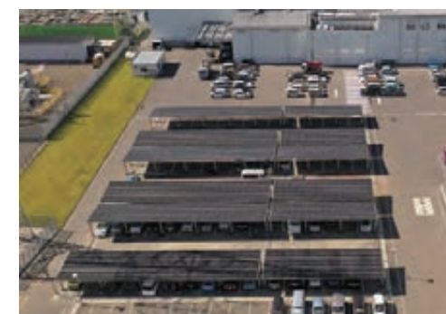
Solar panels at Aoki Foods
