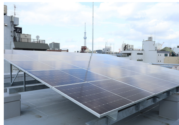
Solar panels on the roof of the Head Office building
