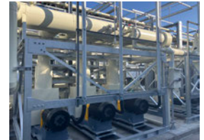
Chilled water system for air conditioning
