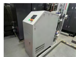
Heat collection system
