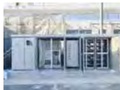
Self-consumption storage battery system
