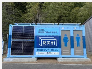
Installed at the disaster-resilient roadside station “Tajima no Mahoroba.”
