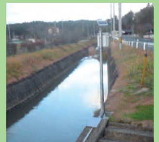
Water level gauge installed in a river
