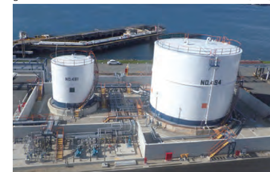
Storage tank for next-generation aviation fuel (SAF)
