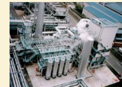
Large-scale hydrogen production facility
