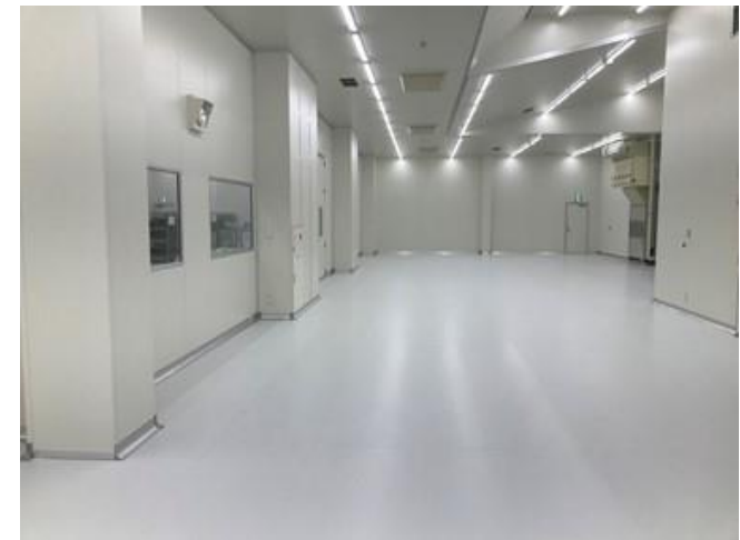
Technical building: Clean room
