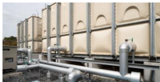
Air conditioning equipment
