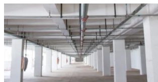
Fire protection equipment
