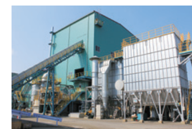
Incineration ash melting furnace facility
