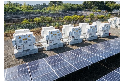
In-house solar power plants operated under FIP conversion + storage battery co-location
