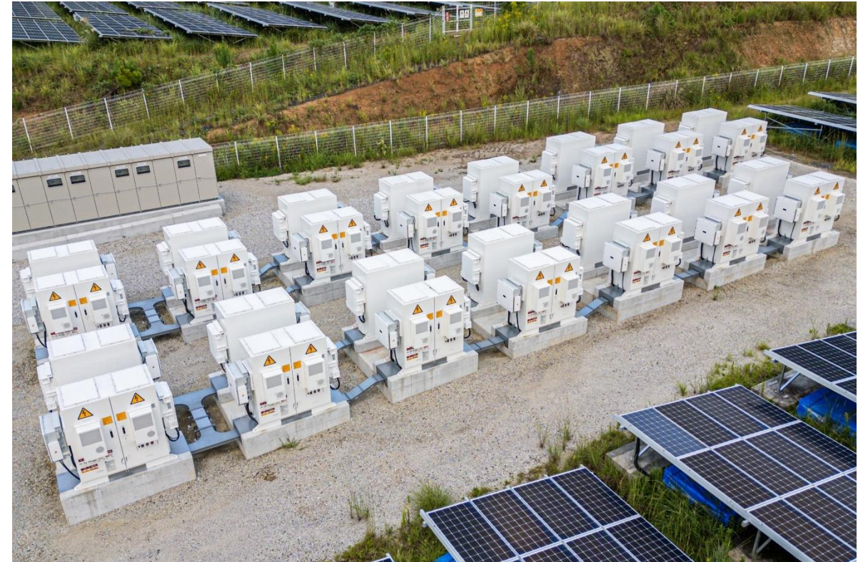
Storage batteries co-located with solar power plant
