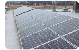
Solar power plants
