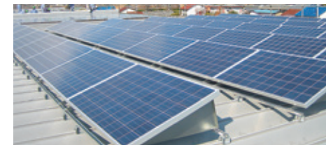
Solar power generation equipment
