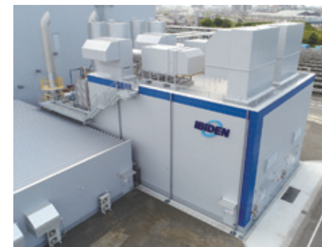
Cogeneration system (Ogaki Central Plant)
