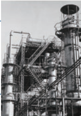
Trichloroethylene production facilities
