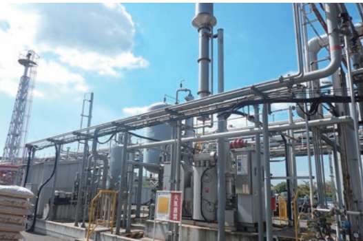
Hydrogen boiler facility at Mizushima Plant
