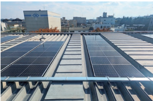
Solar power generation facility at Shibukawa Plant
