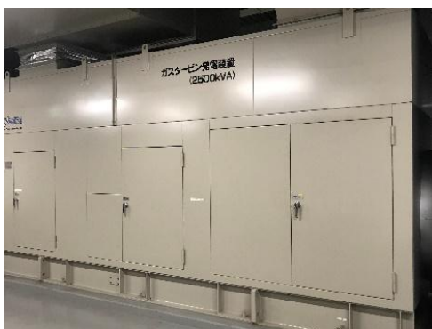
Emergency power generator
