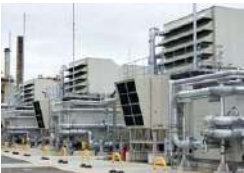
Gas Cogeneration System
