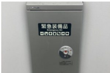
Elevator Disaster Prevention Cabinet
