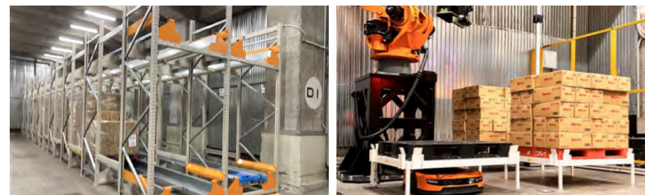
Examples of equipment installed in the R&D Center: Pallet shuttle racking system (left) and palletizing arm robot working with AGVs (right)
