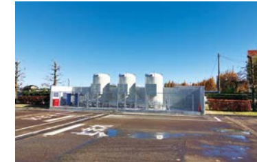
Boiler fuel conversion at our Hokuriku Plant
