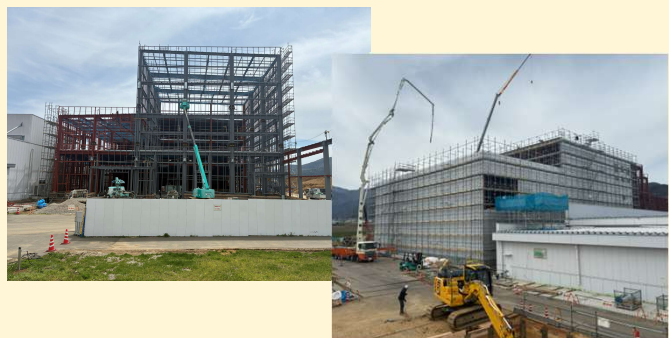
Asahi Plant – Current status
