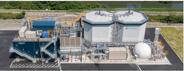
Western Kumamoto Biogas Power Plant
