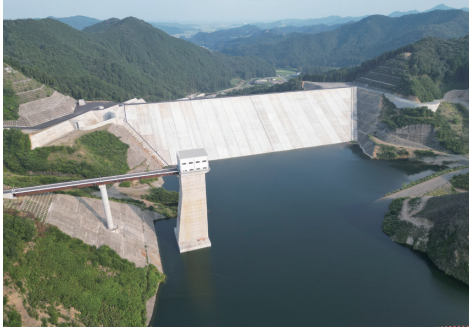
Construction of the Nanma Dam's Primary Structure (Kanuma-shi, Tochigi) Owner: Japan Water Agency
