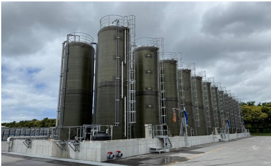
Storage tank terminal completed in the Sodegaura area
